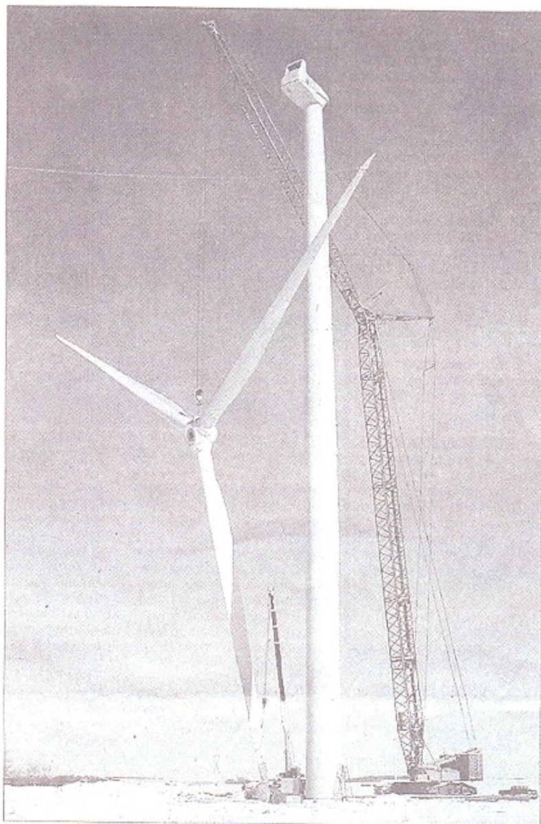
Construction of the St. Leon Wind Project, located about 200 kilometres southwest of Winnipeg, is being managed by GreenWing-Algonquin Power.
